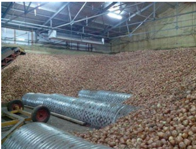
Example of bulk storage pile of potatoes with ventilation piping beneath.
